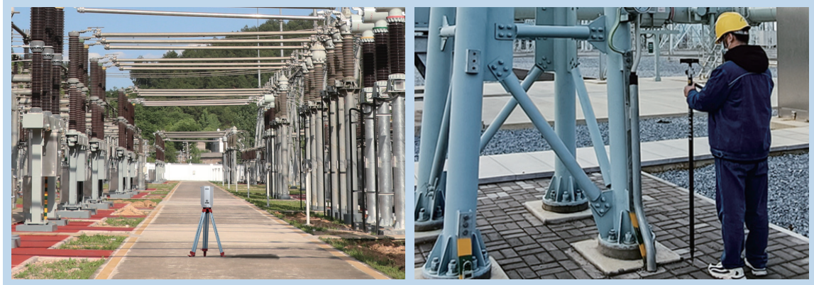
Substation data acquisition FIG4
